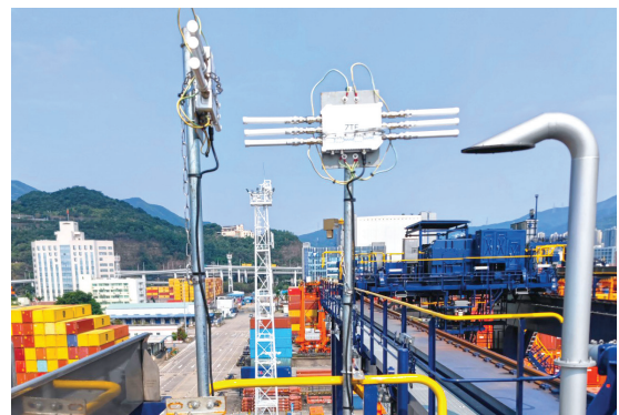
5G network technology installed at YANTIAN.
